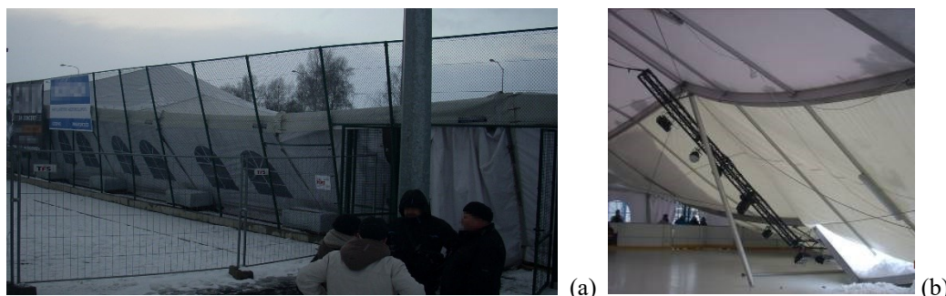
Fig. 3. Disaster of tent hall laden with snow a) external view, b) damaged aluminum girders of ice rink roof in Szczecin, photo PINB Szczecin (public domain) [45]
