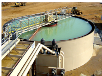
Fig. 11. Installation for thickening beneficiation waste
