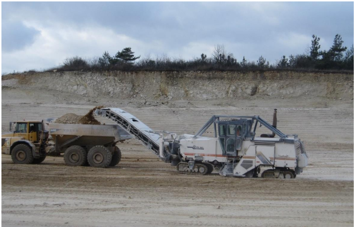
Fig. 1. Operation of the Wirtgen 2200 SM combine with direct loading onto technological trucks on the "Raciszyn" limestone deposit.
