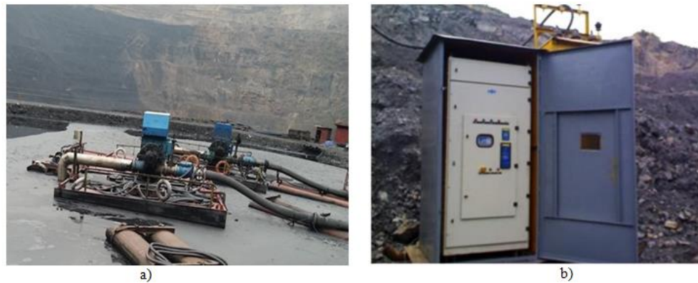
Fig. 4. Power supply of a mine water pump motor in Vietnam: a mine drainage pump (left) and a conversion device (right).
