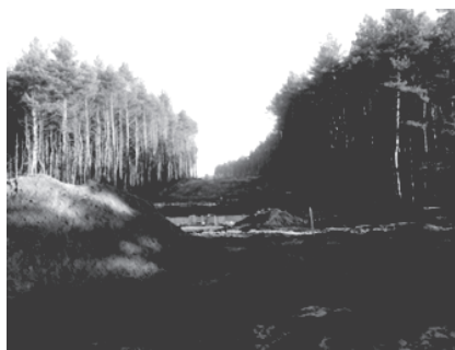
Fig. 2. Construction of the motorway around Olkusz (Poland) Interference with the natural environment (deforestation) (Photo by M. Gomułka)
